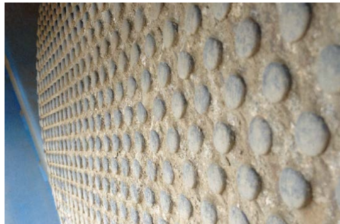
Figure 15 - Wear lining condition ~1,000 hrs in service (courtesy of AngloGold Ashanti)
